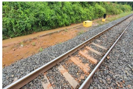
(b) Kondisi Mud Pumping
