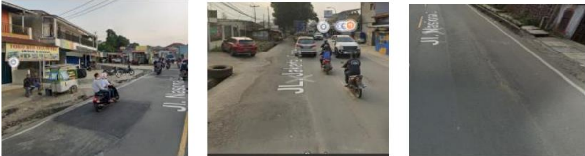
Figure 2. Road Damage Mapping Results Using Google Street View Map
